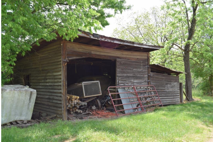
Equipment shed and chicken house at the Miller House, east and north elevations
